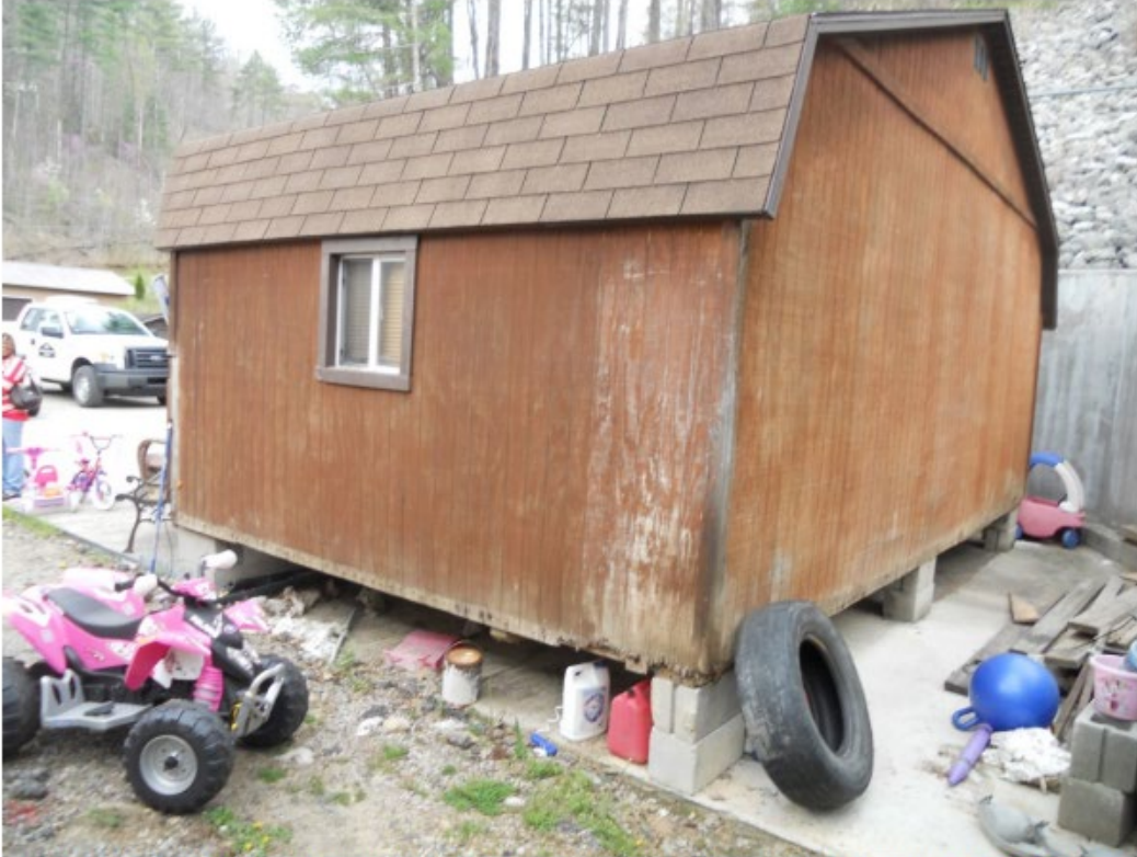
Storage shed being used as a home for mother and children. Building is not connected to water, sewer or electricity (using and extension cord).
